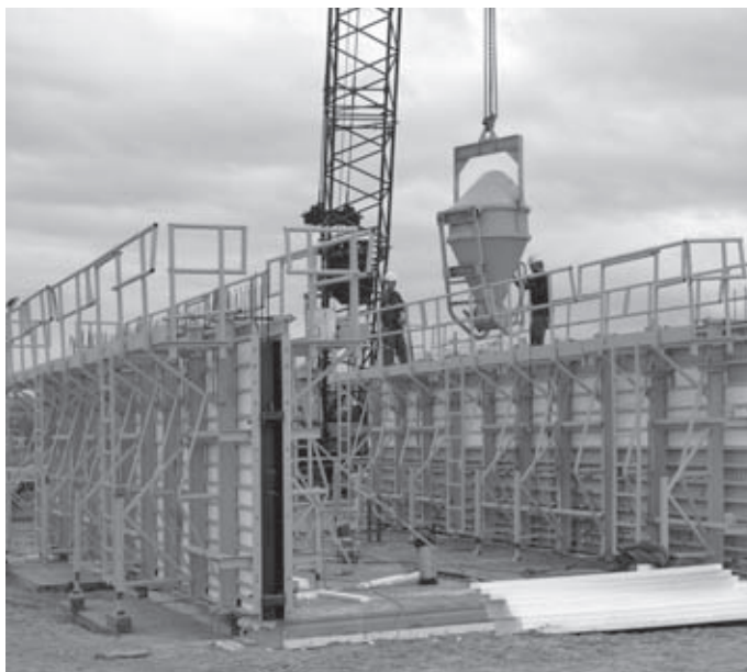
Tunnels storten in Almere
